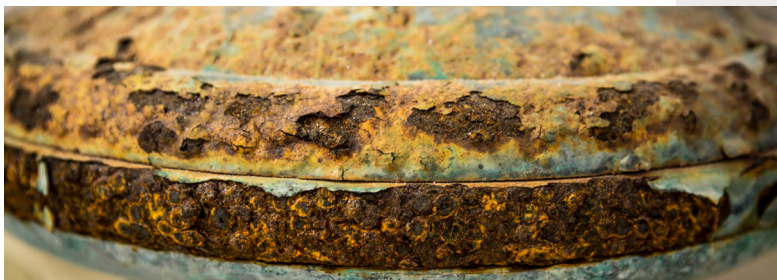
CORROSION OF AN OUTDOOR FIXTURE
